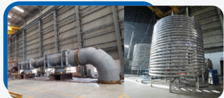
Critical Power / Process Piping & Coils
